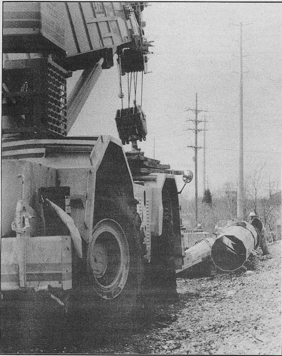
Construction on power lines continues, despite protest by the community of Webster Groves.
