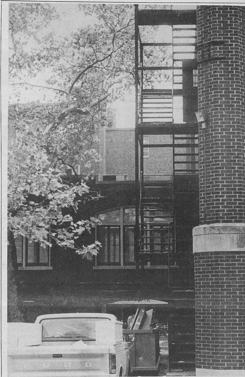
Loretto Hall's fire escape, part of the student protection system found to be safe, by Webster and city standards. Photo: Kim Helfrich
