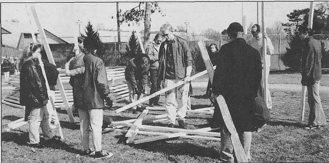
Students from Tim Curtis' 3D design class spends a Monday afternoon constructing centralized modular units for an upcoming project.
