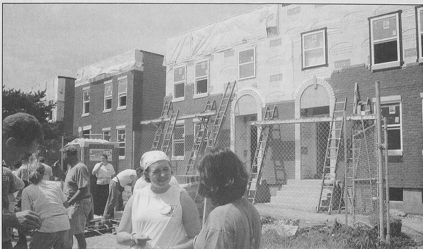
Volunteers from Webster University stand in front of several of the 22 homes the St. Louis chapter of Habitat for Humanity is building. The homes are located in mid-town St. Louis, off of Grand Avenue. BARB SETTLES / Contributing Photographer
