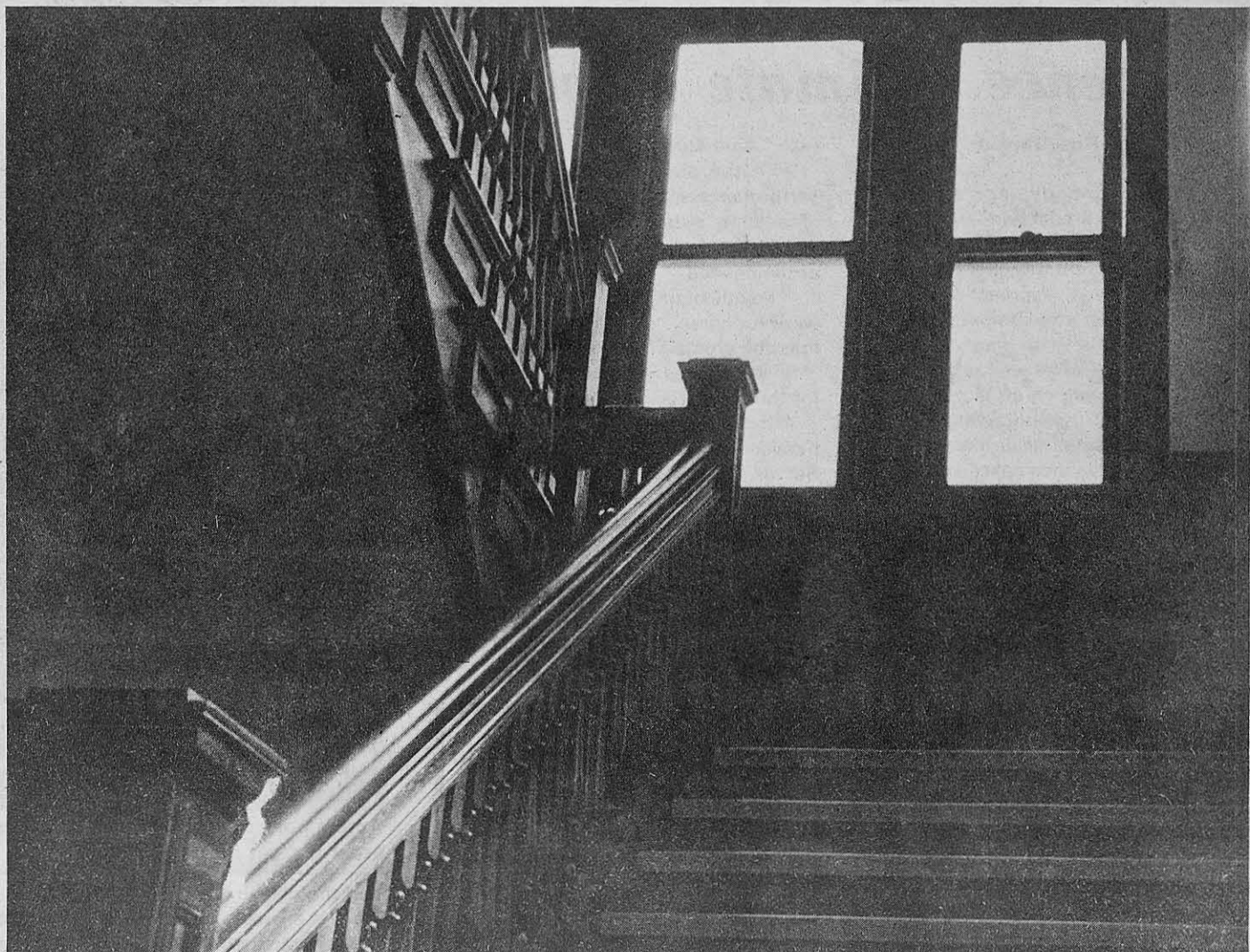
An empty stairway leading to the 4th floor: This is a problem to many when the elevator is in disrepair.
