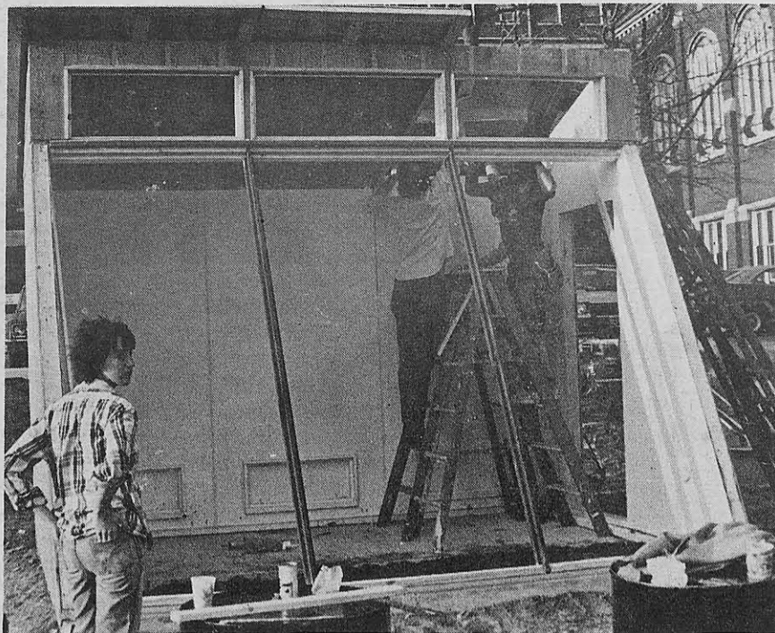
The roof goes up on the new solar greenhouse, which stands on the old tennis courts. photo by Brian Schaff
