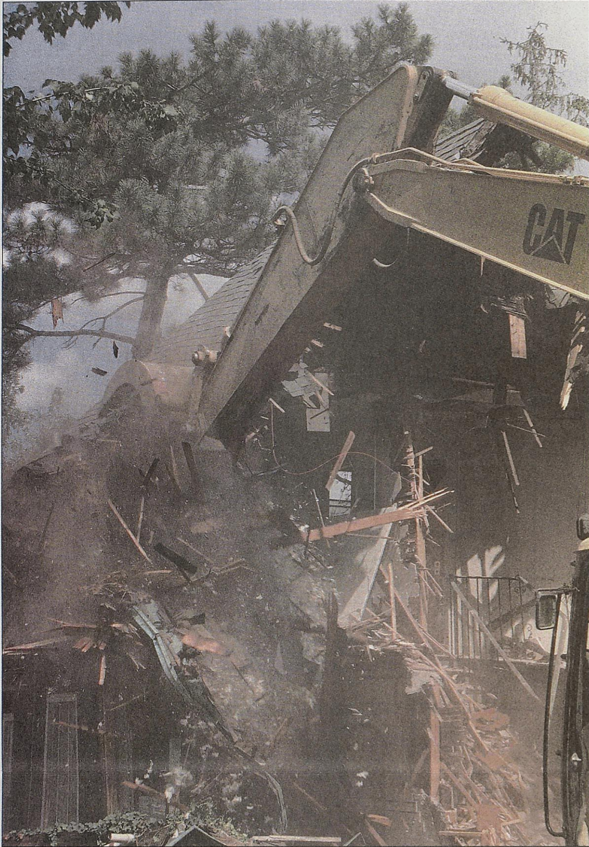
Debris flies as half of the Brown House still stands.
