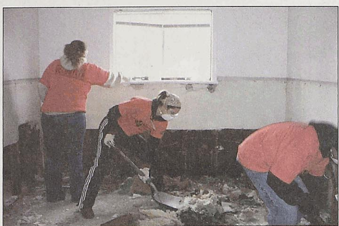
PHOTO COURTESY OF SANDY BUSKEN Sandy Busken (center) shovels debris March 29 while Cate Cearley (left) and Mario Santander continue to gut a home damaged by floodwaters from the Meramec River in Pacific, Mo.
