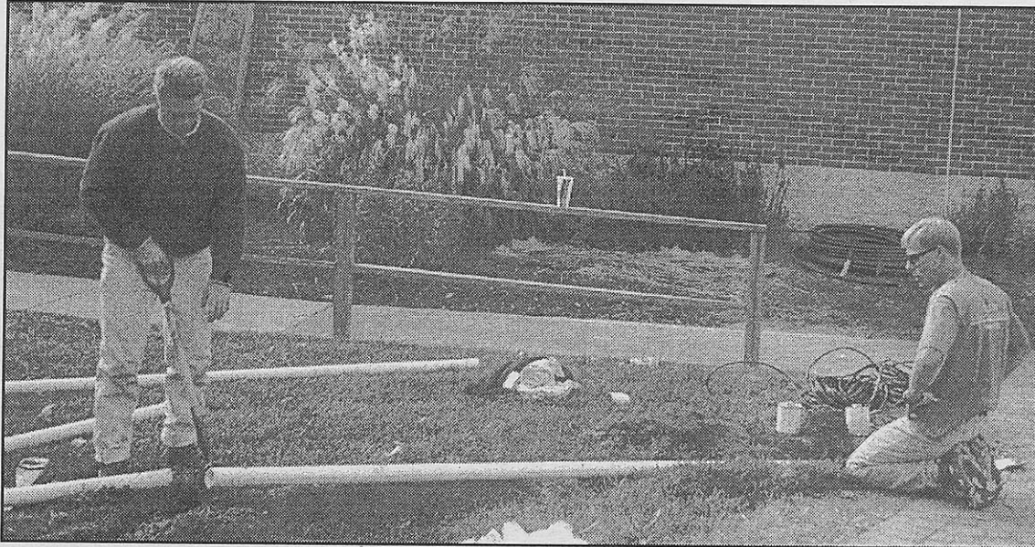
Phillip Boschert, left, and Eric Valentine install inground sprinklers in the quad Oct 23. Boschert and Valentine work for Allen Irrigation & Lawn Care, Inc.
